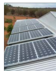
Solar array, Mt Peachy, Central Australia
