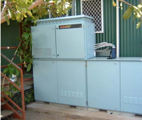
Bushlight has recently installed the first of the new generation of Bushlight Household RE Systems at Galawdjapin, Northern Territory
