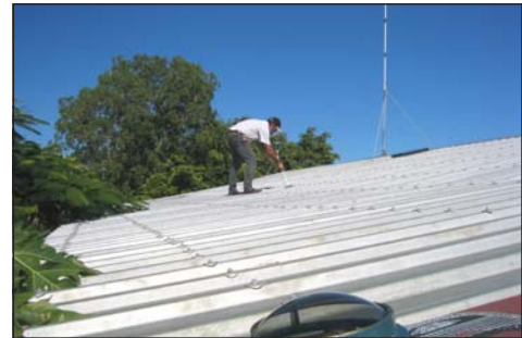
Using a Solar Pathfinder to check the roof orientation for possible future PV array location - Gunun Woonun
