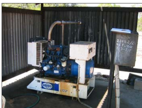
Typical large diesel generator used in many outstations
