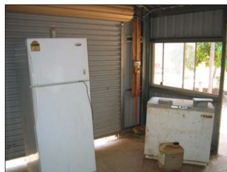
Using a diesel generator to keep this fridge and freezer cool for one day could mean that some communities are spending up to $26.00 a day on 20 litres of diesel.
