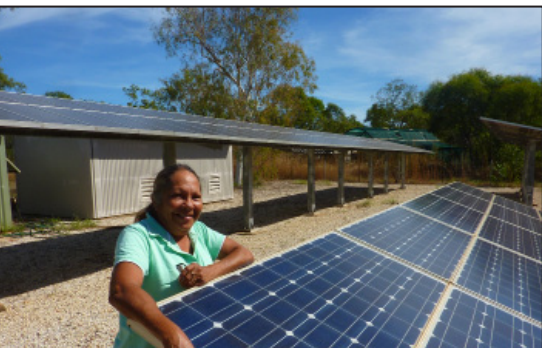
Roma Puertollano and the Bushlight solar array
