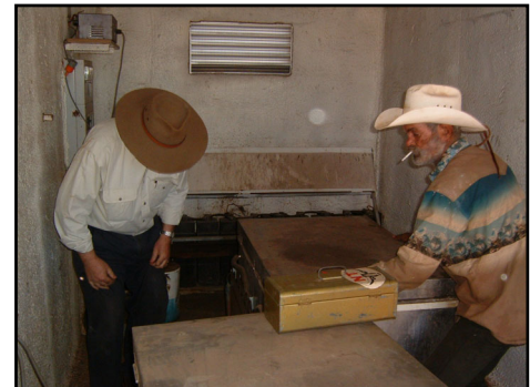
Bushlight Regional Manager NWWA, John Schmidt, examines an old DC freezer with community leader, Brian Dann at Ngarantjadu
