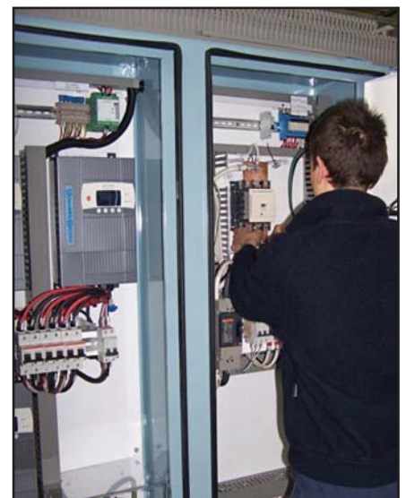
Factory testing of the new enclosure
