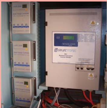
The charge controllers and inverter at Paradise Farm, Kakadu are monitored from the office in Alice Springs
