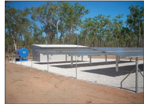
The Bushlight Hybrid RE system at Kapalga
