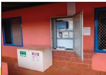
The new equipment enclosure is easier and safer to access
