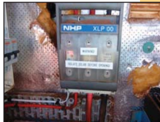
The insulation was deteriorated
