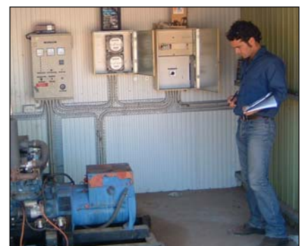
Assessing a generator – Ben Purcell, Bushlight Central Australia
