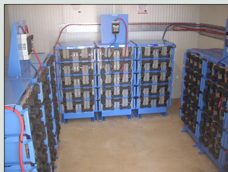
The battery bank at Ulpanyali
