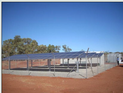
The Bushlight solar array at Ulpanyali
