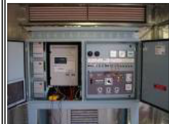
Ukaka's Bushlight System being commissioned
