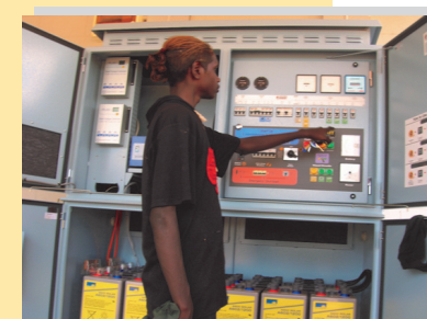
Learning about the main system control enclosure, Gurungu (Elliot), Northern Territory, October 2006.
