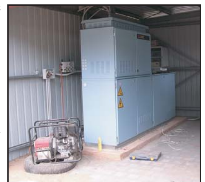
Equipment and battery enclosures at Wumajbarr
