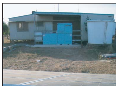
Household RE system installed at Gubbanguru in June 2005
