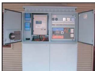
Community system enclosure with PS 1-6 Inverter
