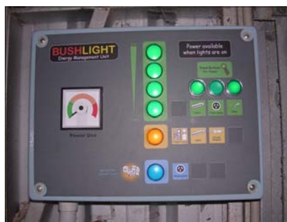
Bushlight's Energy Management Unit
