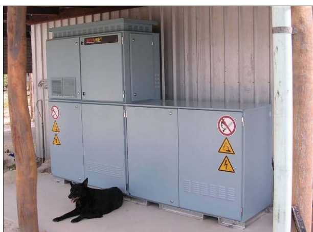
The installed Household RE System
