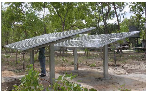
Free standing solar array
