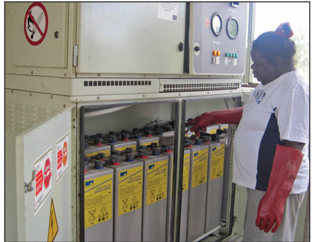
Selma Hoosan cleaning cobwebs from the gel cell batteries on a Bushlight system during training
