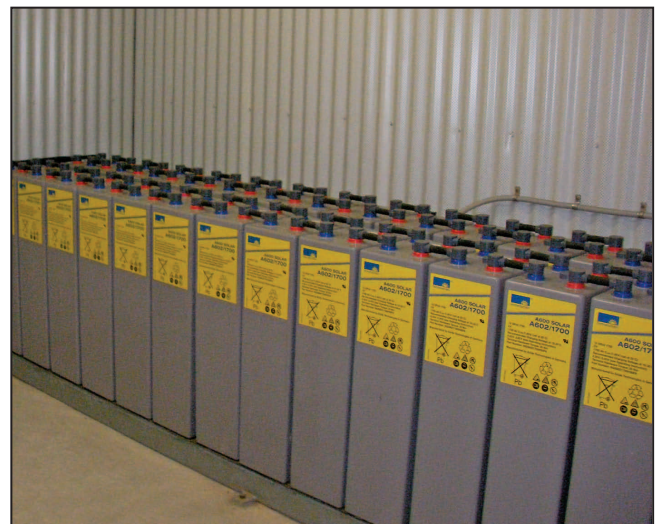
A typical Bushlight RE system battery bank
