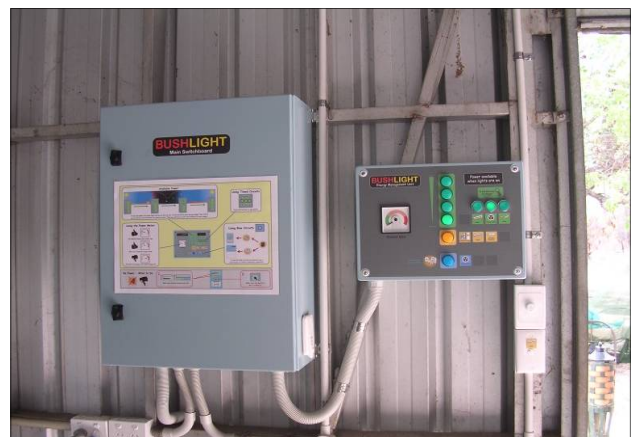
The Energy Management Unit and Switchboard in the main shed
