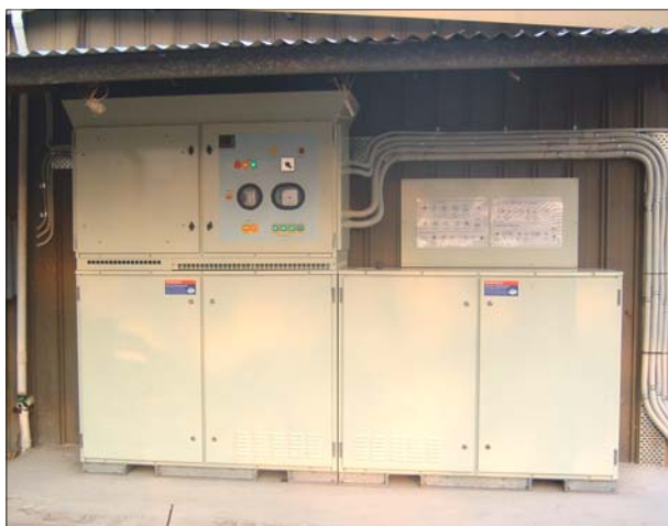
The Bushlight household RE system at Dingo Spring
