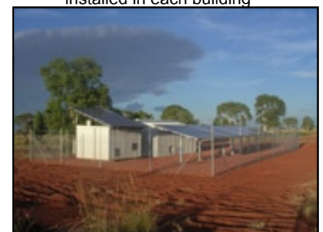
The new Bushlight RE system at Mt Theo
