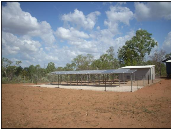
The upgraded Bushlight system with addition panels at Wandigalla
