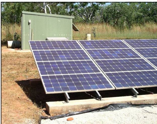
The pre-existing solar array at Chile Creek
