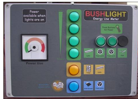
Bushlight Energy Management Unit
