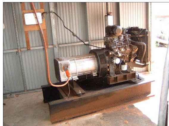
Blue Bush's generator is now used very rarely
