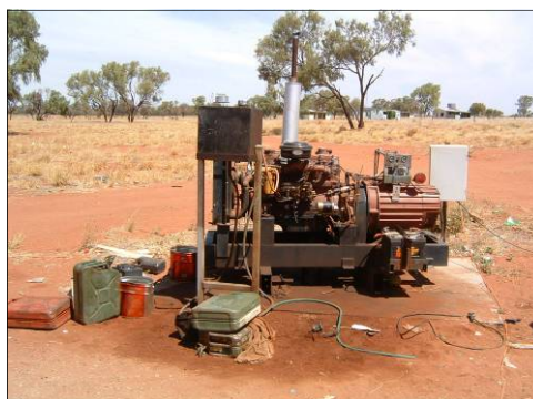
Prior generator at Irrerlirre
