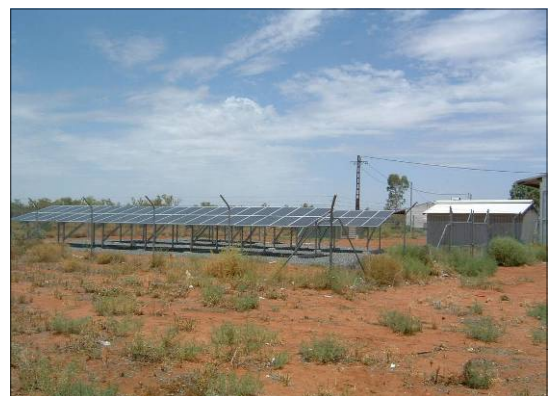
Bushlight array and shed at Irrerlirre
