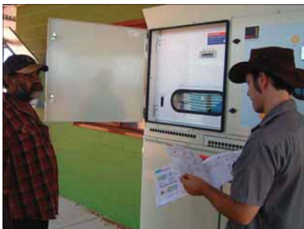
Ben Purcell of Bushlight provides training in the use of Bushlight RE Household System to Bob Palmer at Corkwood Bore
