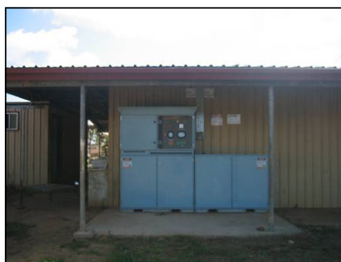
The system is located under the rear existing verandah.
