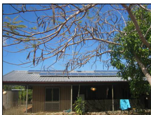
The PV arrays for the system are roof mounted.
