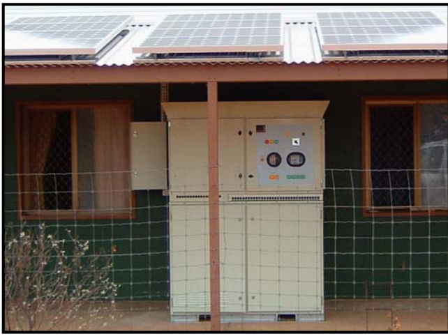
The New Bushlight Household System was commissioned on 26 th December 2003
