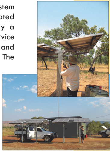
Non-Bushlight systems in the Kimberley being reviewed for inclusion in the Maintenance program.
