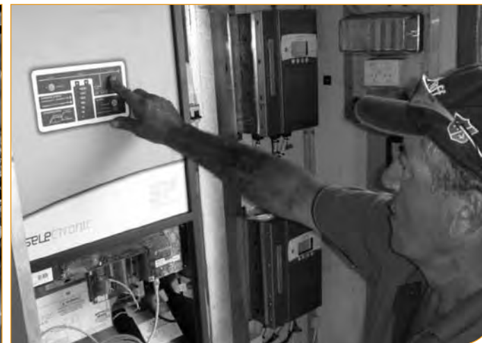
Users being trained to operate the CAT Bushlight RE System.
