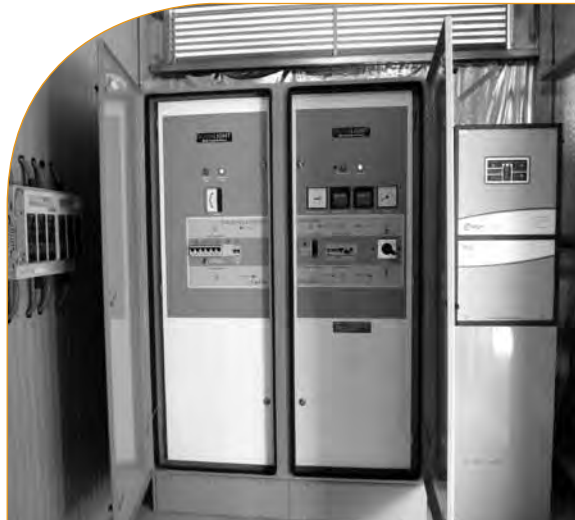
Bushlight's award winning stand-alone power system at Raymangirr, NT.
