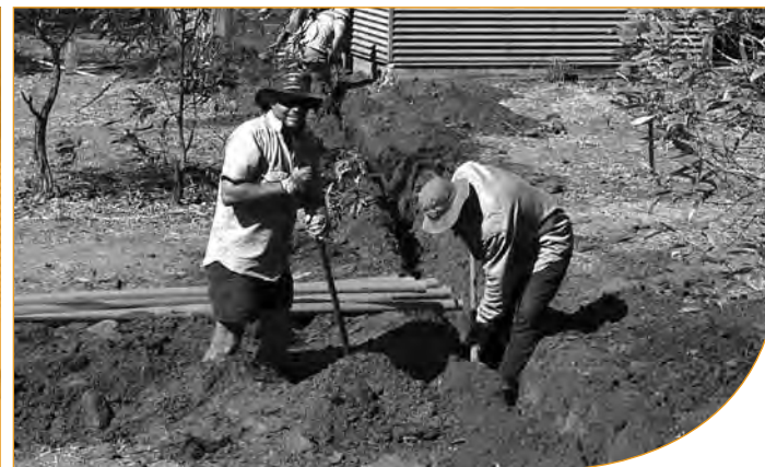
Electrical contractors from Gully's Electrical, part of Bushlight's RE Electrical Contractors Network. Photo courtesy of Glen Parker, Gully's Electrical.
